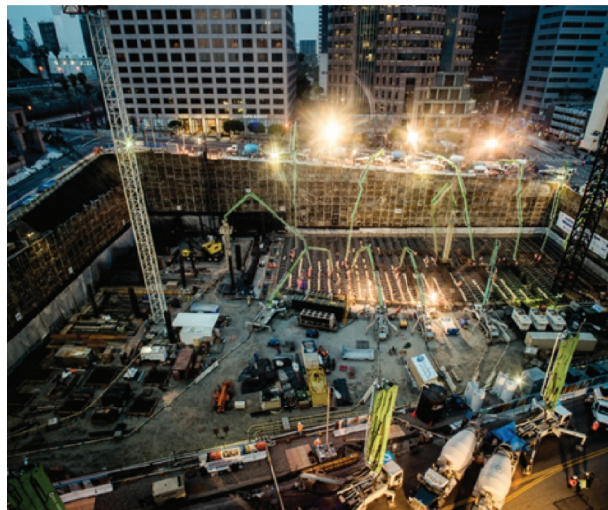
Vulcan supplied nearly 32,000 tons of aggregates in less than 24 hours for the February 16, 2014 world record-setting foundation pour for The Wilshire Grand Center in downtown Los Angeles.
